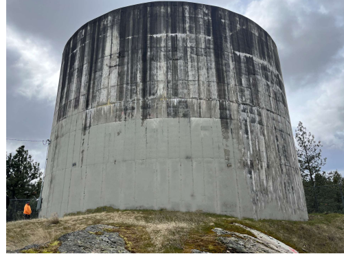
1.2 MG Storage Tank
